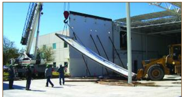
The crew uses a crane and bulldozer to lift one of the wall panels.
